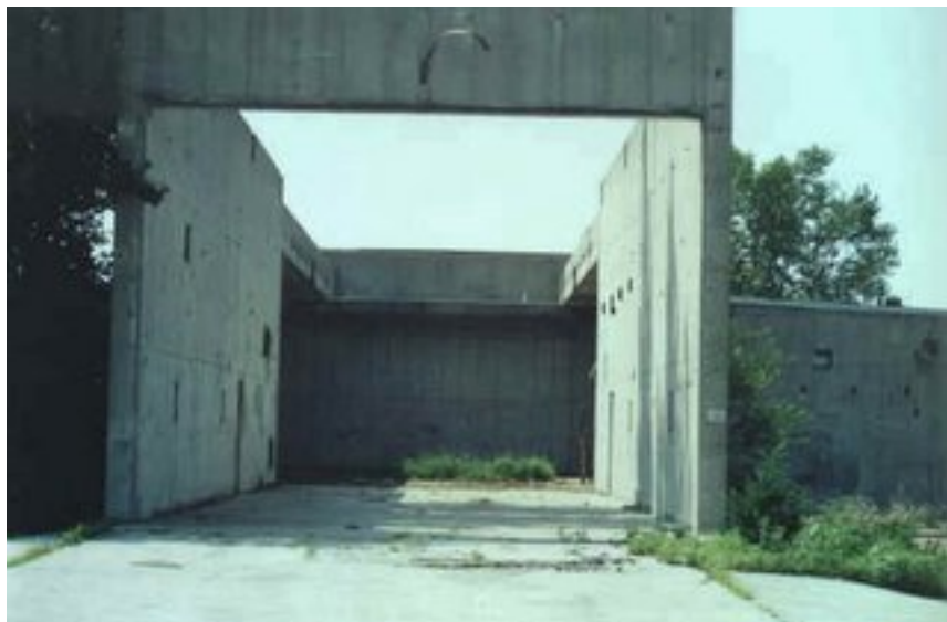
This is the command center entrance, back in 1962 this would have been a classified complex.
